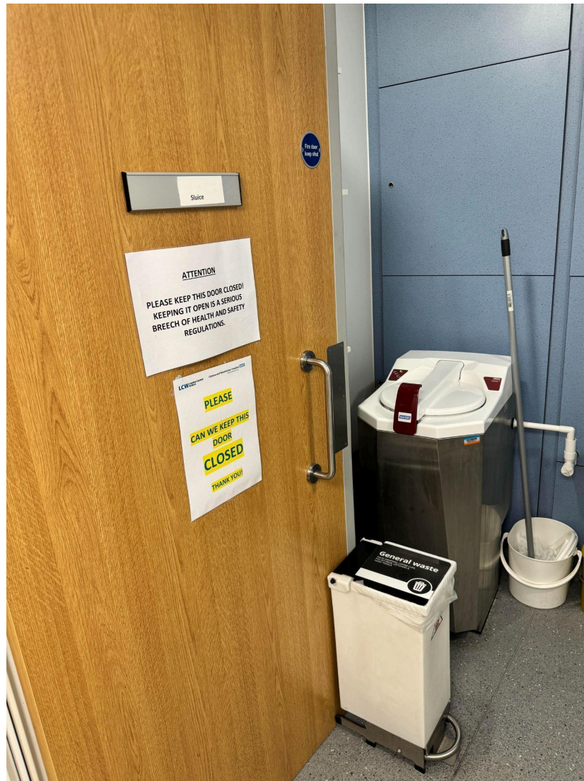
Figure 5. Door to sluice in the UTC being propped open, despite a sign asking to keep the door closed.
